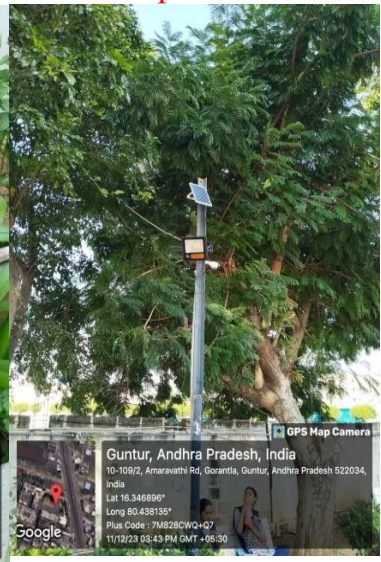
Solar lamp stands-50volts
