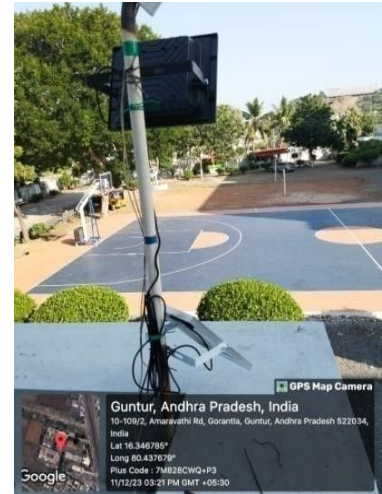
Solar lamp stands-50volts
